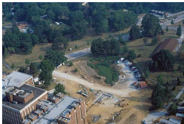
Aerial view of Bugg Lake after it had been drained for the construction of the Research Building
