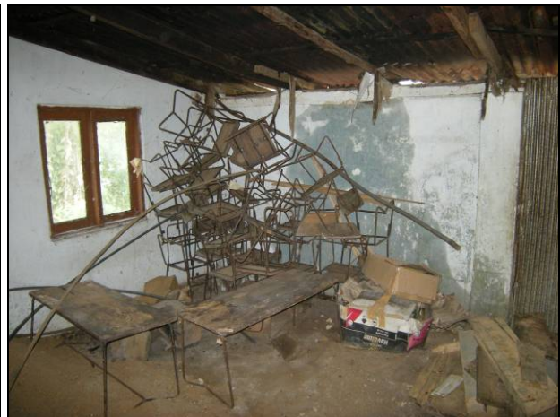
Computer Room Site
